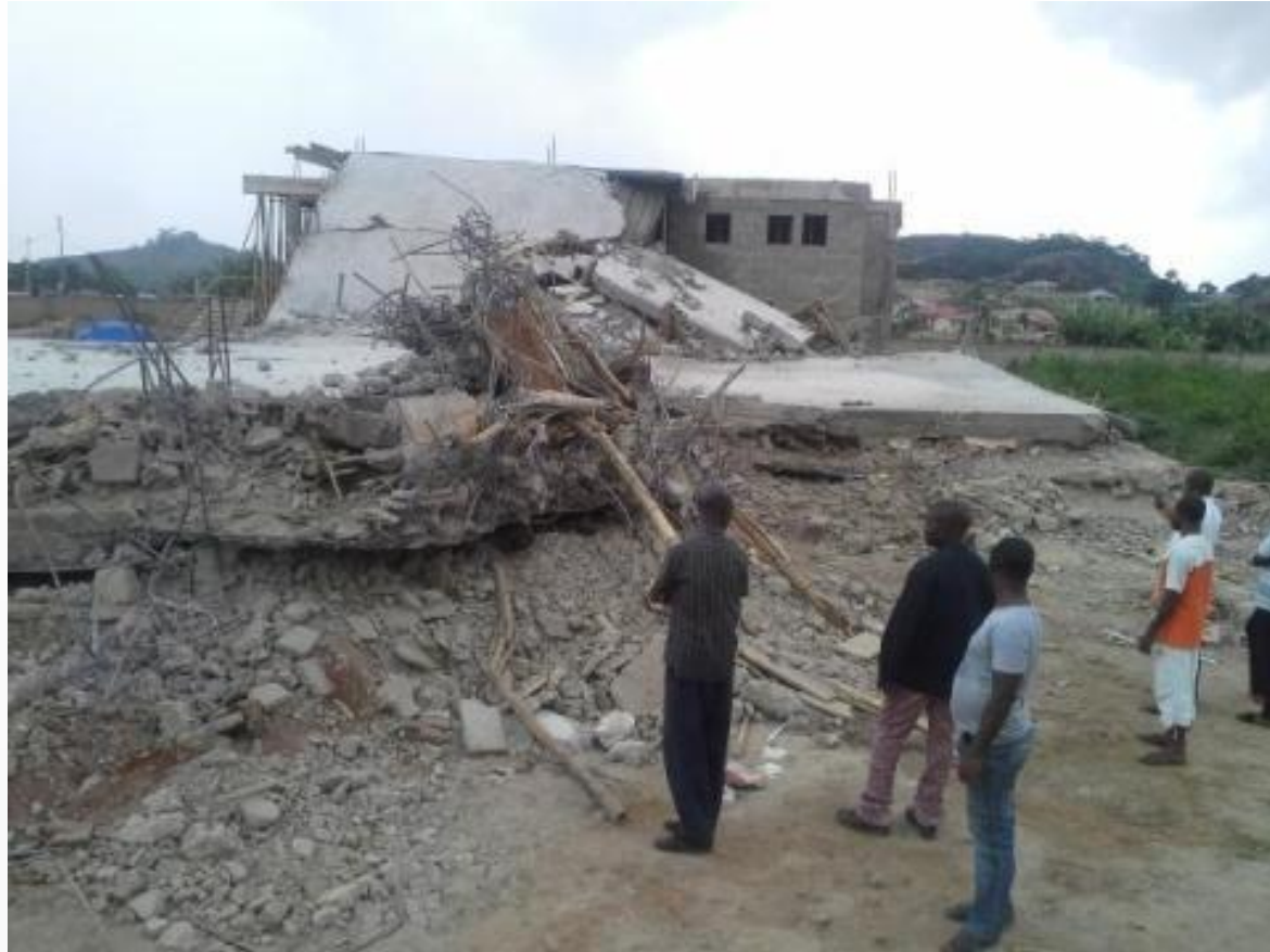
Plate V: An uncompleted storey building belonging to Homaj private secondary school at Igoba community in Akure North local government area of Ondo State – May 7, 2014
