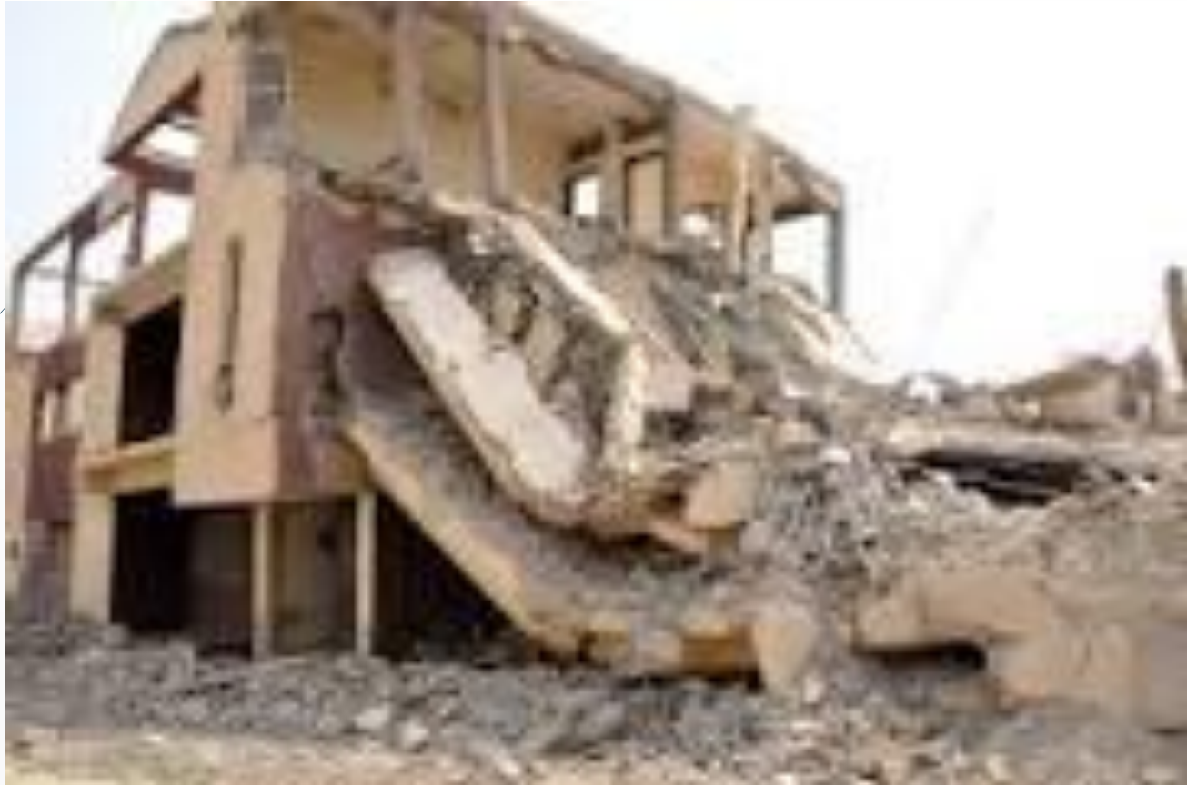
Plate I: Partial Building Collapse at Gwarinpa (45 th Road, 1 st Avenue), Abuja – 12 th January, 2012
