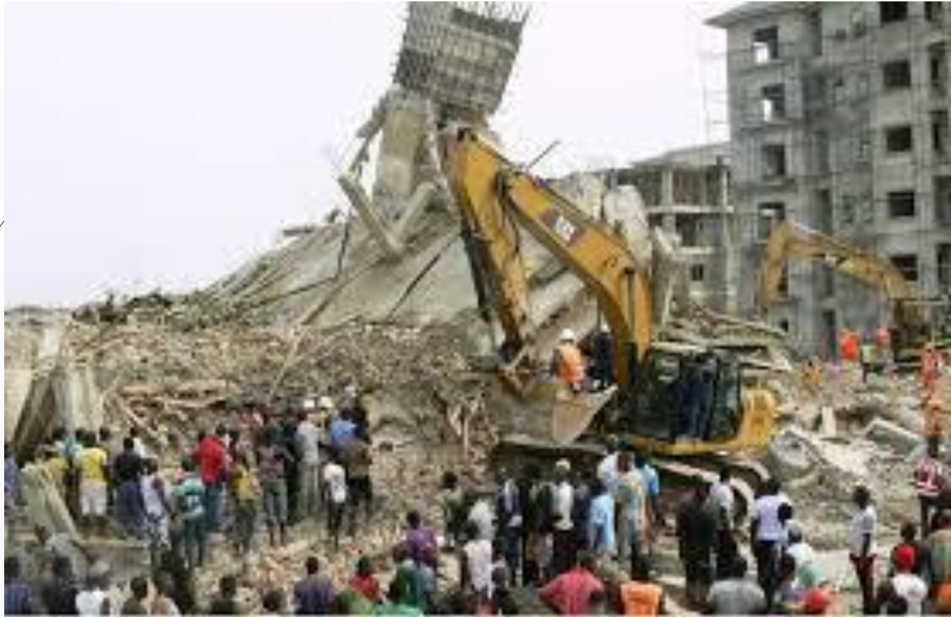
Plate IV: 6 Storey Synagogue Hostel Building Collapse that Claimed 116 lives – 12 th September, 2014, Ikotun, Lagos.
